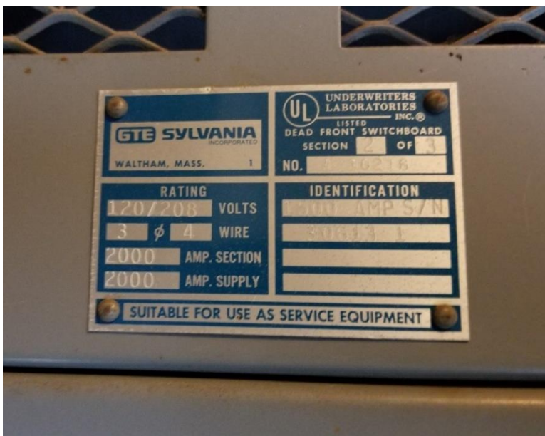
Figure 18: Main Panel 2000A, 120V/208V Servicing Clubhouse 5
