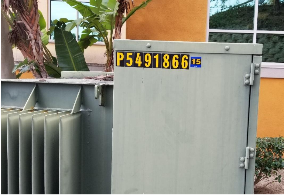
Figure 25: SCE 1500kVA 277/480V Pad-mounted Transformer Servicing the Community Center
