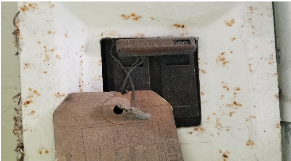
Figure 10: One of the Main Breakers for a Residential Panel at C219
