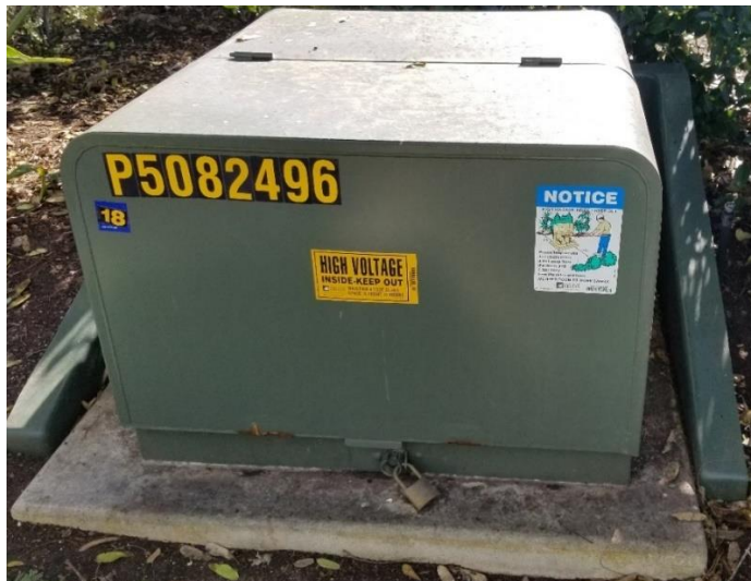
Figure 20: SCE 75kVA 120V/240V Pad-mounted Transformer Servicing Clubhouse 6
