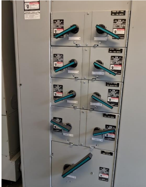
Figure 12: SCE 800A 277/480V Panel Servicing Clubhouse 2
