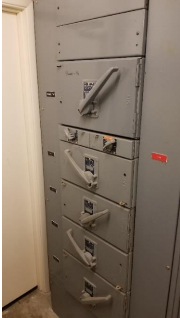
Figure 16: Main 2000A 120/208V Switchgear Servicing Clubhouse 4
