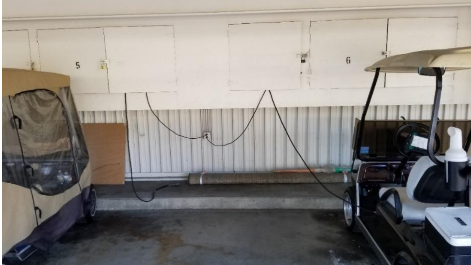
Figure 7: Example of Golf Cart Charging via Battery Charger in Storage Cabinet Plugged into Outlet
