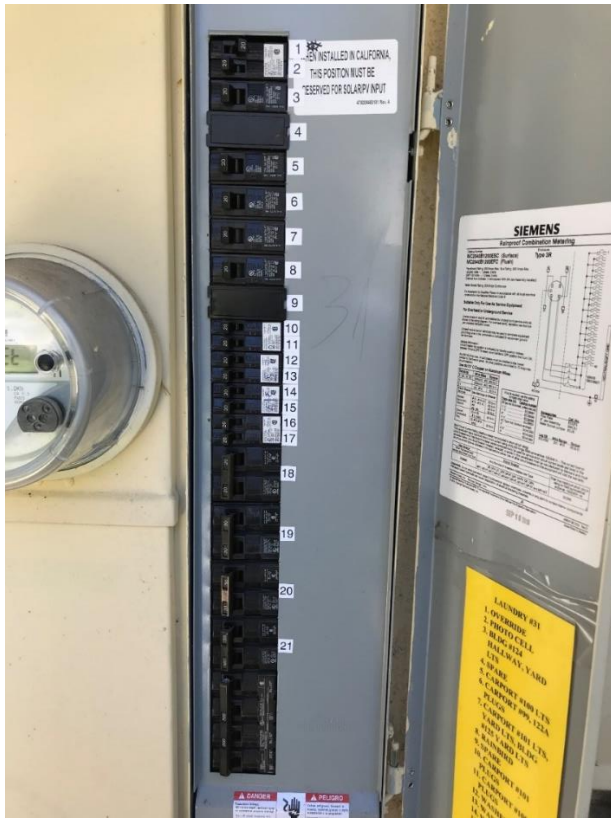
Figure 13: New Subpanel Servicing Laundry Room 31
