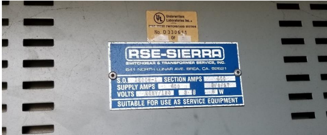
Figure 28: 400A 120/208V Main Panel Servicing the Library
