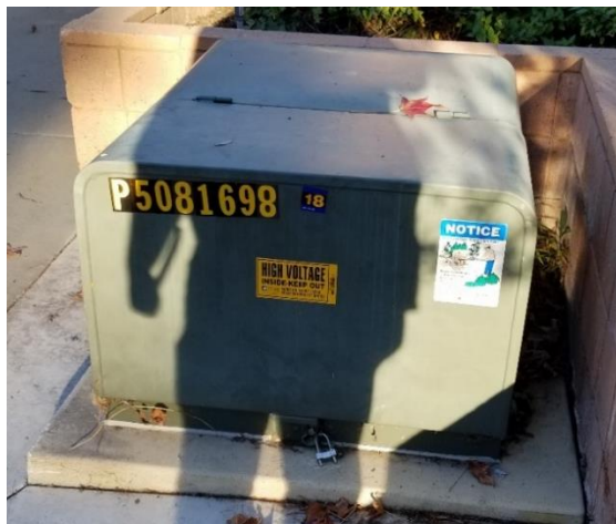
Figure 15: SCE Transformer at L142
