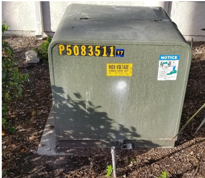
Figure 8: Pad-Mounted Transformer Servicing a Third Laguna Hills Mutual Residences at C219
