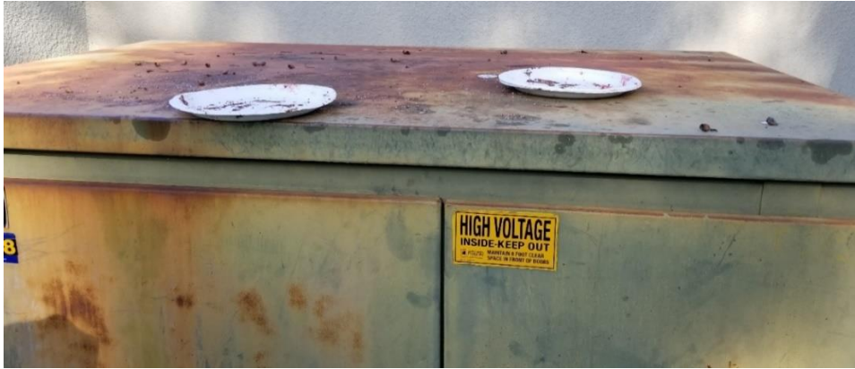
Figure 17: SCE 300kVA 120V/208V Pad-mounted Transformer Servicing Clubhouse 5
