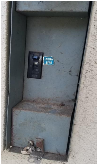
Figure 16: Laundry Room 226 Main Breaker Panel in Laguna Hills Mutual Residential Area
