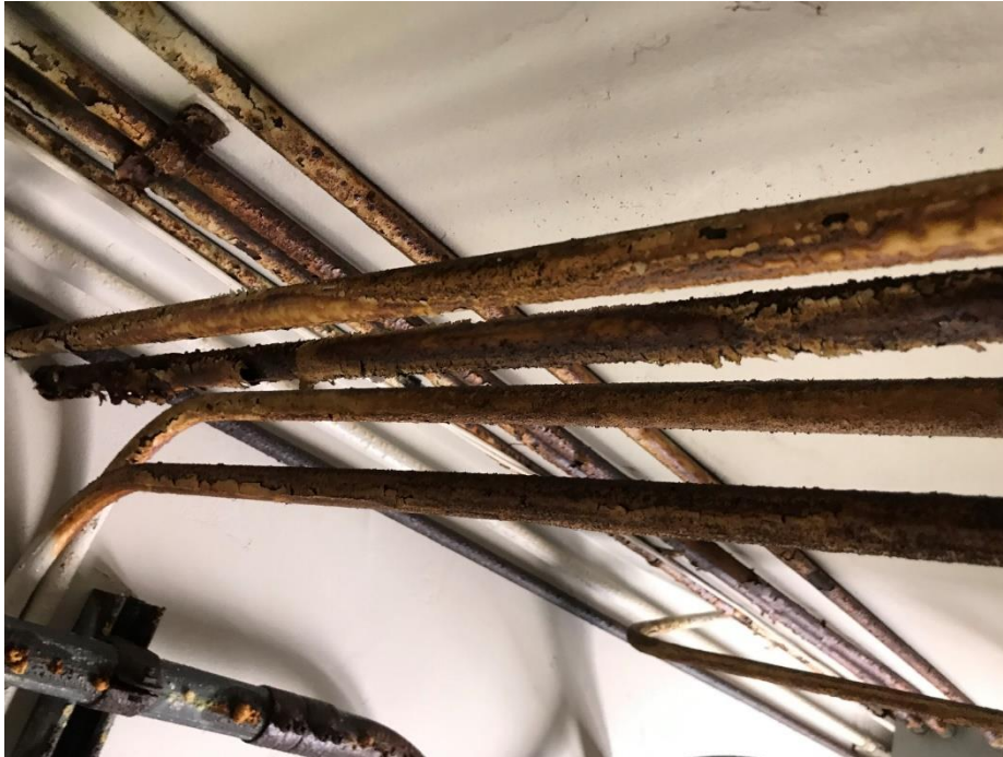
Figure 6: Corroded Piping Found in Clubhouse 1 Main Electrical Room
