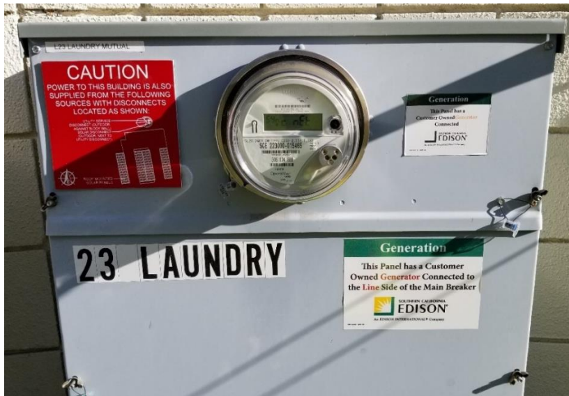
Figure 11: Solar Electric Supply Servicing Laundry Room 23
