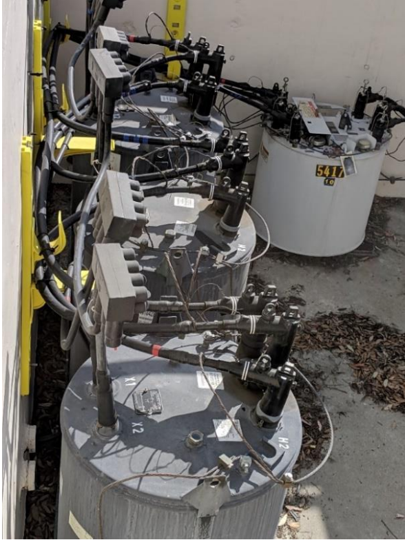
Figure 11: SCE 3-100kVA 120V/208V Overhead Transformer Servicing Clubhouse 2
