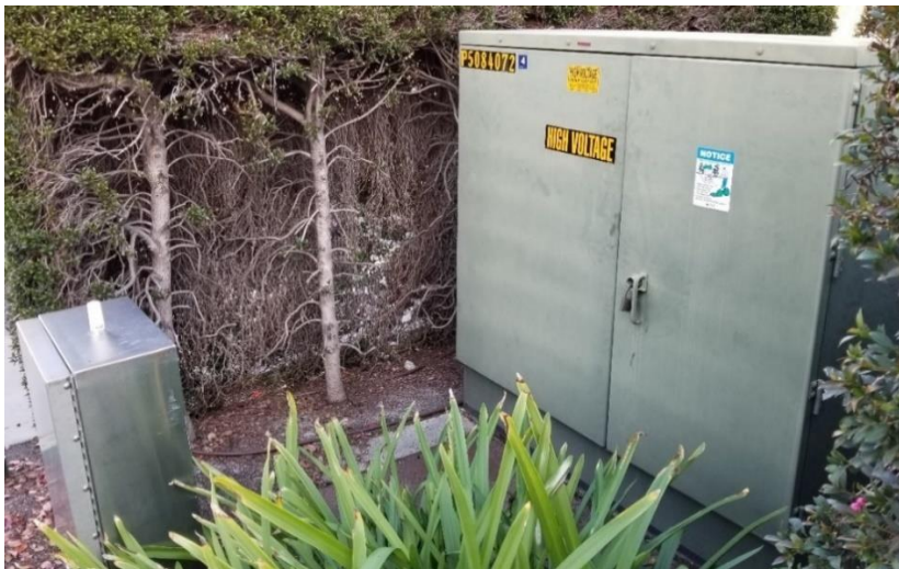
Figure 13: SCE 500kVA 120V/208V Pad-mounted Transformer Servicing Clubhouse 3
