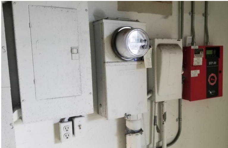
Figure 17: 480V Panel Servicing a Third Laguna Hills Mutual Elevator at C219
