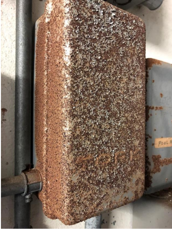
Figure 22: Rusted Junction Box Servicing Clubhouse 6
