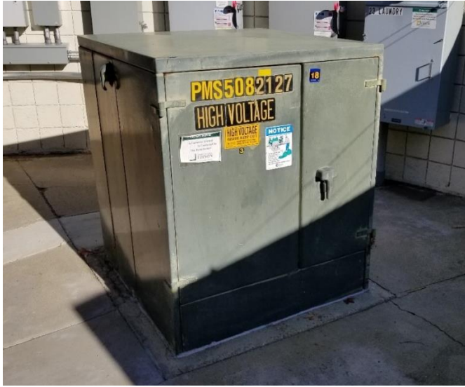
Figure 10: SCE Transformer Servicing Laundry Room 23
