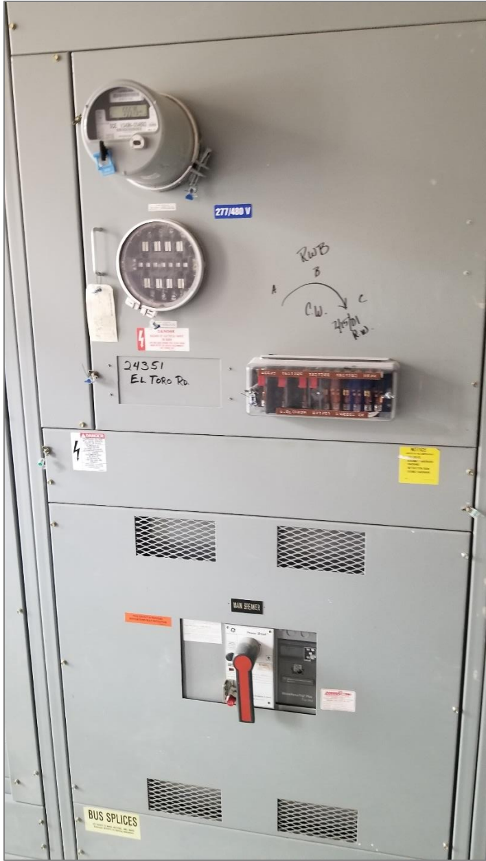
Figure 26: 2000A, 277/480V Main Switch Serving the Community Center
