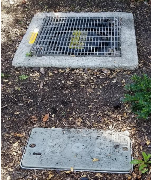
Figure 6: Typical Subsurface Transformer Servicing a Laguna Hills Residential Area
