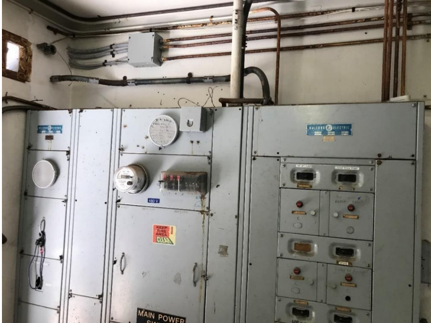
Figure 7: Electrical Switchboard and Meter Found in Clubhouse 1 Main Electrical Room
