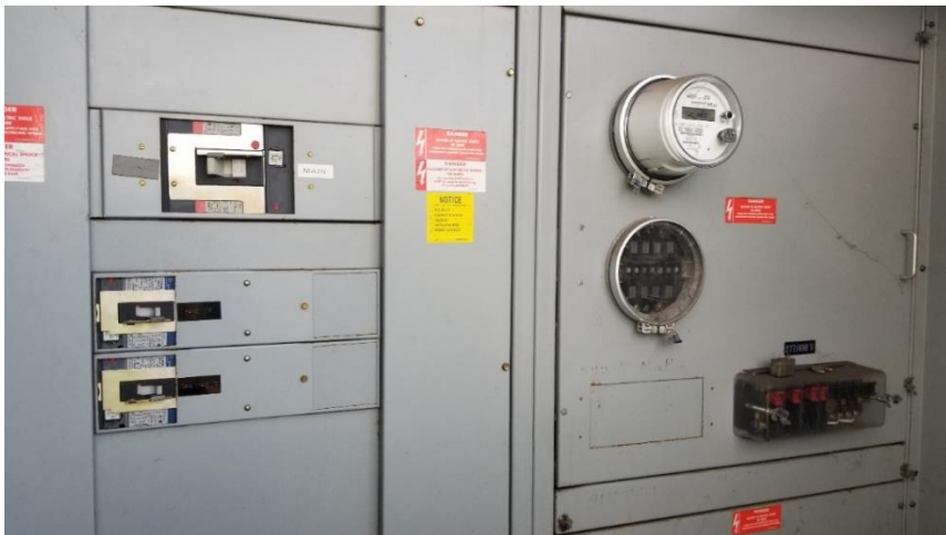
Figure 24: 400A 277/480V Main Panel Servicing Clubhouse 7
