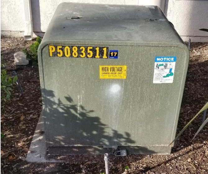
Figure 5: Pad-Mounted Transformer Servicing a Third Laguna Hills Mutual Residential Area (C219)
