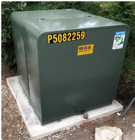
Figure 7: Pad-Mounted Transformer Servicing Laundry Room 90
