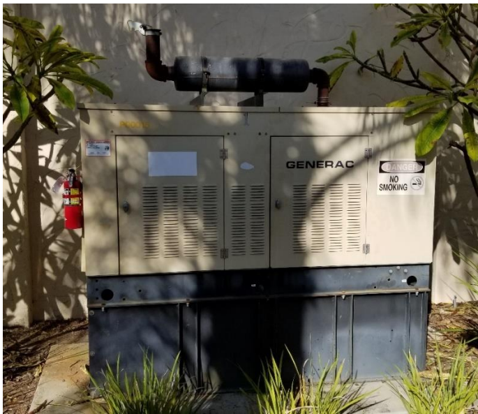
Figure 10: Diesel Backup Power Generator at Clubhouse 1
