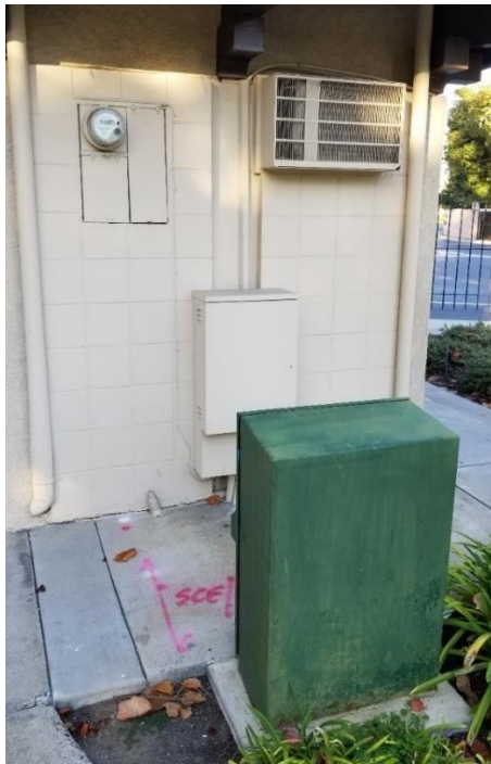
Figure 29: 60A 120/240V Main Panel Servicing Gatehouse 2
