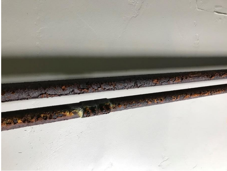
Figure 9: Corroded Conduit Changed Out Four Years Ago Found in Clubhouse 1 Main Electrical Room
