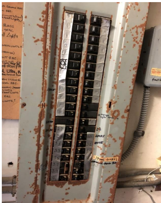
Figure 21: Rusted Breaker Panel Servicing Clubhouse 6
