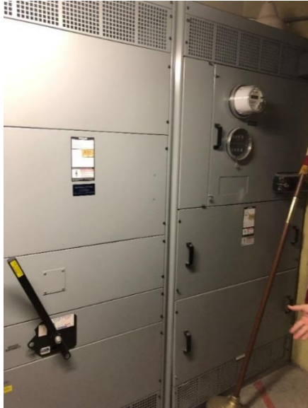
Figure 14: Main Panel 1600A, 120V/208V Servicing Clubhouse 3
