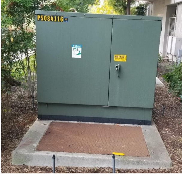
Figure 16: Pad-mounted transformer servicing a Third Laguna Hills Mutual Elevator at C219
