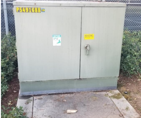
Figure 23: SCE 300kVA 277/480V Pad-mounted Transformer Servicing Clubhouse 7
