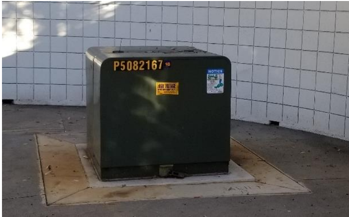
Figure 5: Pad-Mounted Transformer Servicing a United Laguna Hills Mutual Residential Area
