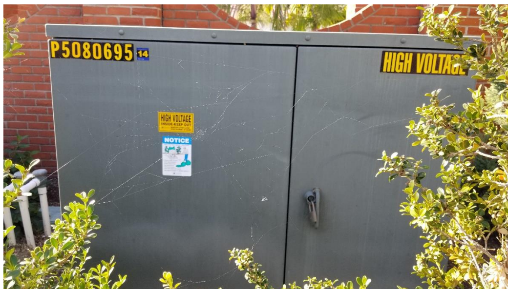
Figure 5: SCE 225kVA 120V/208V Pad-mounted Transformer Servicing Clubhouse 1
