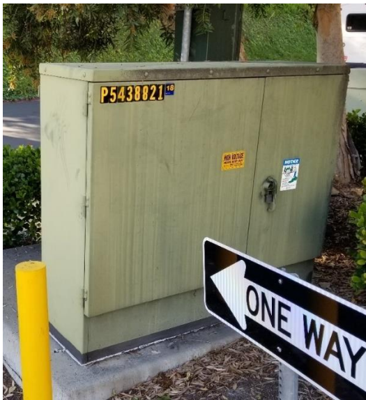
Figure 27: SCE 75kVA 120/2080V Pad-mounted Transformer Servicing the Library
