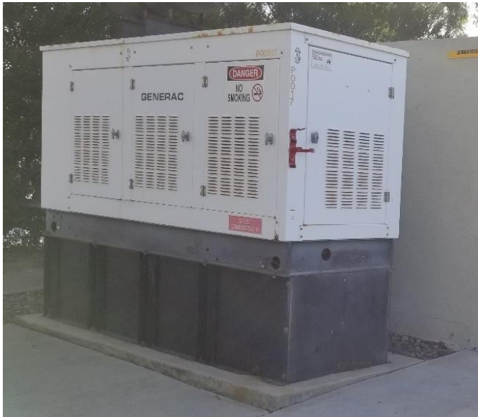
Figure 19: 194kVA Emergency Generator Servicing Clubhouse 5
