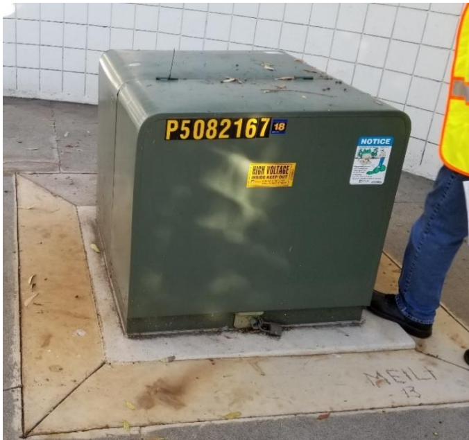
Figure 12: SCE Transformer Servicing Laundry Room 31
