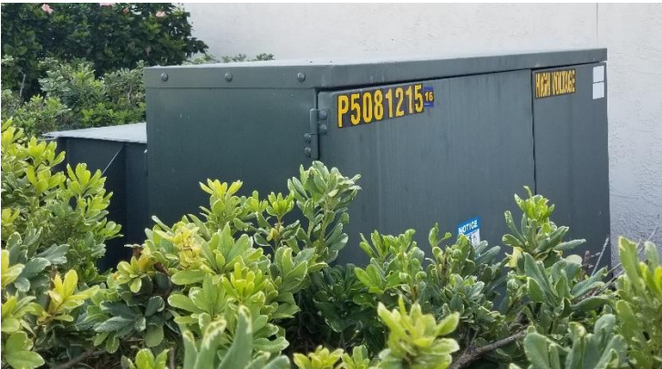
Figure 15: SCE 300kVA 120V/208V Pad-mounted Transformer Servicing Clubhouse 4
